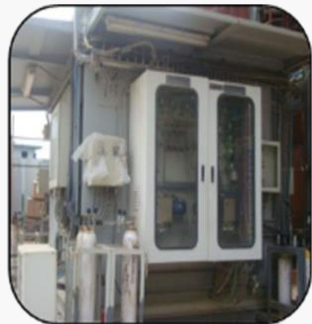
CEMS at Calciner
