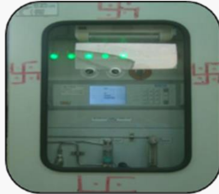
CEMS at Power Plant
